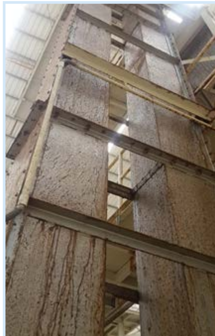
Closed system - cannot be cleaned
